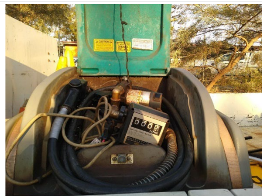
The secured fuel pump compartment with meter readings gauge, but no gauge dip or access for a dip stick to measure stock level to detect fuel theft.
