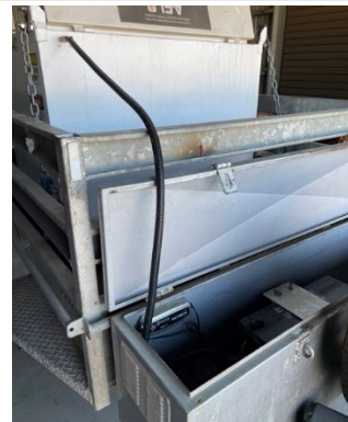
A separate secured compartment to store the battery and cable to operate the fuel tank. The cable is put away after use in the secured compartment.
