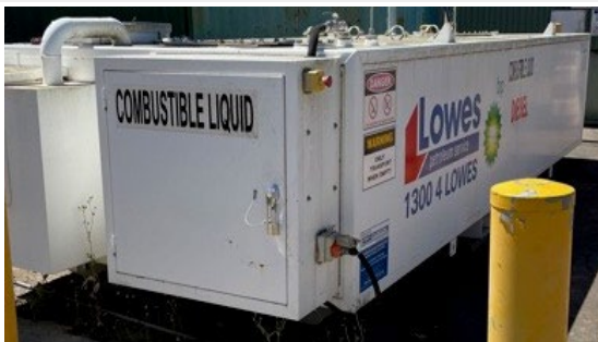
Figure 2: Bulk fuel tank (10,000L) including features
