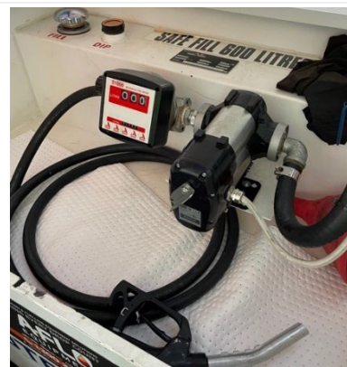
The secured fuel pump compartment with meter readings gauge.
